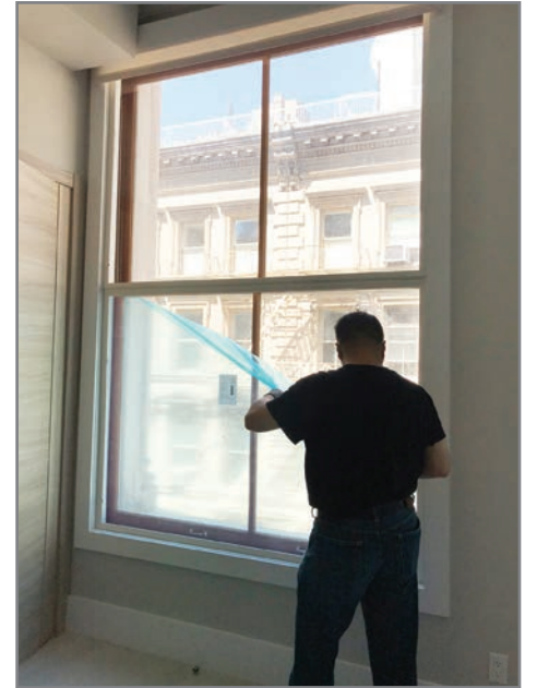
A new insert being placed into a window frame in a historic building
